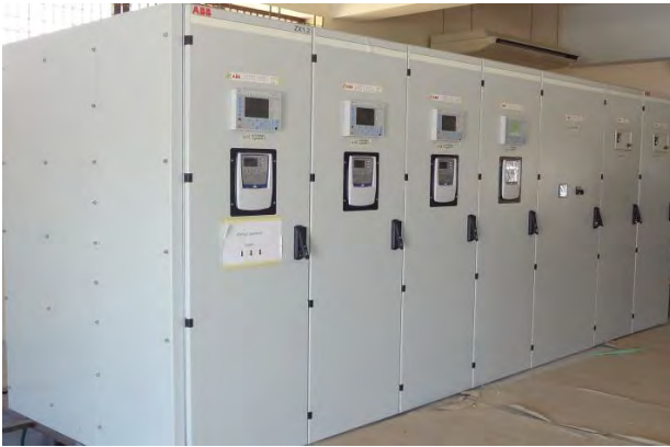
33 KV GIS Switch Gear at IEPZ, Ishwardi, Pabna.
