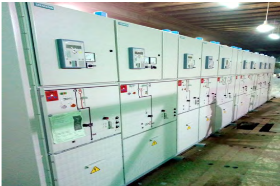
33 KV GIS Switch Gear at National Parliament Bhavan, Sher-E-Banglanagar, Dhaka.
