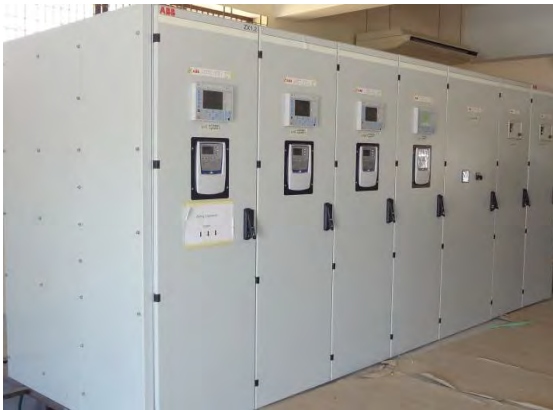
33 KV GIS Switch Gear at IEPZ, Ishwardi, Pabna.
