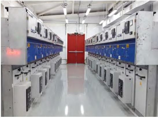
Control Room of 33/11 Sub-station Rooppur Nuclear Power Plant Project, Rooppur Ishwardi, Pabna.
