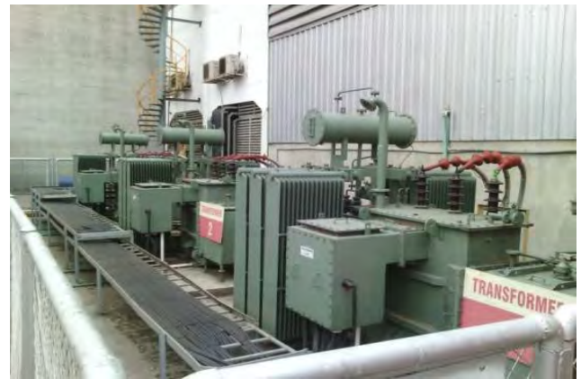
33/0.4 KV, 5 MVA Sub-station at Dhaka Feed Mill Project, Chandra, Gazipur.
