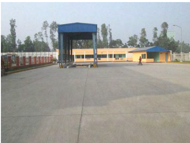
Internal Road/Pavement work, Total Area: 23000 sqm at Chittagong Feed mill Project, Mirsharai, Chittagong
