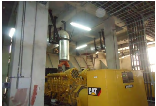
Supply & Installation of 2 MVA Generator at CP Chittagong Feed Mill Project
