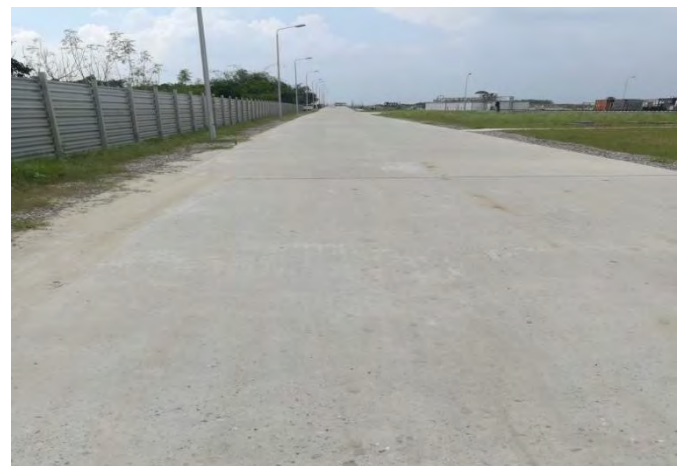
Internal Road/Pavement work at Rooppur Nuclear Power Plant Project, Ishwardi, Pabna, Total area : 52000 sqm
