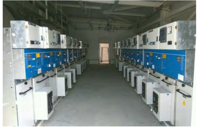
Control Room of 33/11 Sub-station Rooppur Nuclear Power Plant Project, Rooppur Ishwardi, Pabna.
