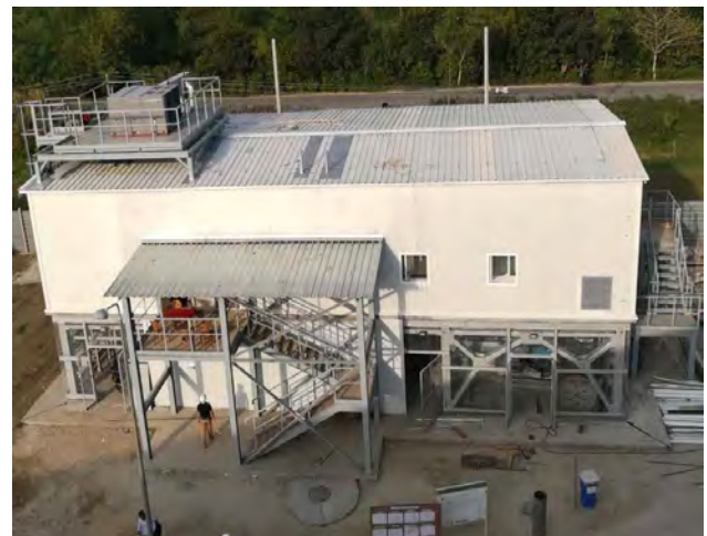
Steel Building for 33/11 KV Distribution Substation At Rooppur NPP Project, Ishwardi, Pabna.
